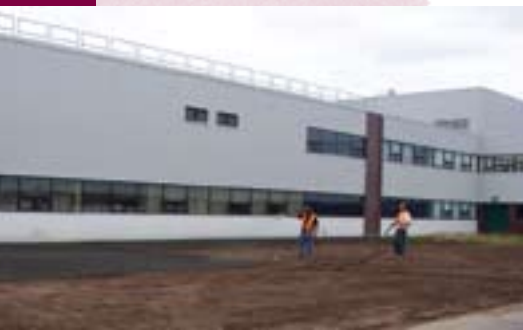
Phase I of construction was completed for renovations at Happy Valley-Goose Bay Campus.
