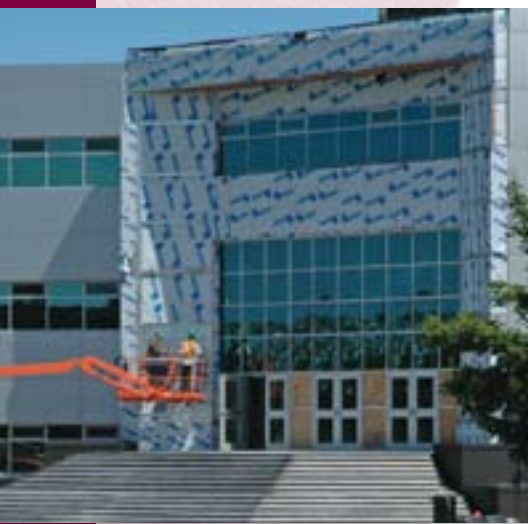
As part of the college's plan to enhance and modernize infrastructure, Prince Philip Drive Campus began many renovations including the installation of a new building envelope.
